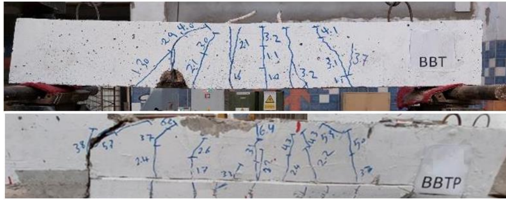
FIGURE 13. The cracking pattern of beams tested in bending until failure
